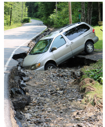
Flood damage in the Stoddard/Alstead area.
